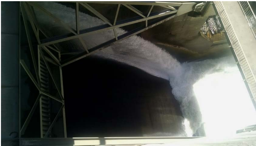
Photo 2. Spillway 1 seal leak while gate is in the closed position.
