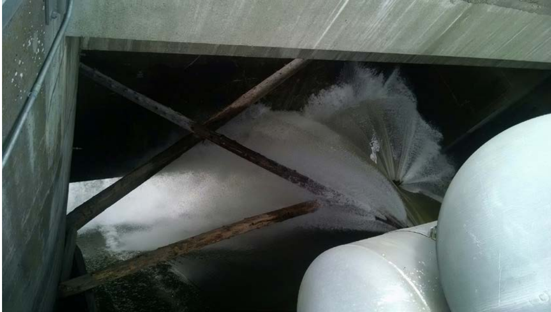
Photo 1. Logs wedged between RSW and spillways gate June 19, 2017.
